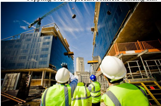
Figure 3.4 Falling Debris, Materials or Objects
