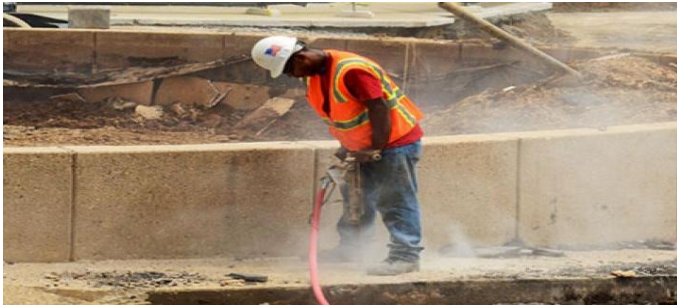
Figure 3.12 Dust causes in construction site
