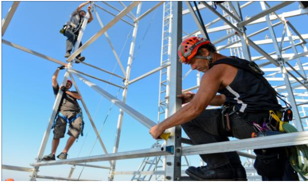
Figure .3.1 fall from High Heights or Scaffolding Causes
