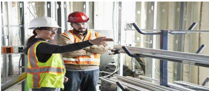
Figure 3.15 Electrical Hazards causes in construction site
