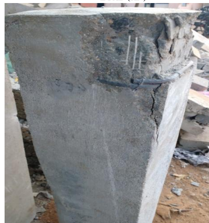
Figure.7. Failure of Scrim Reinforced Column
