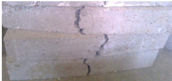
Figure.4. Crack at the bottom of the beam
