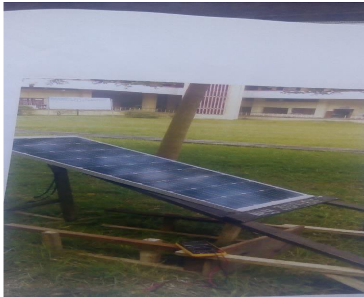
Figure.1. Partially shaded monocrystalline solar module in situ.
