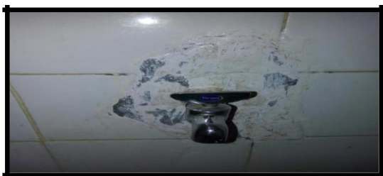
Figure.1. Tiles break while drilling.
