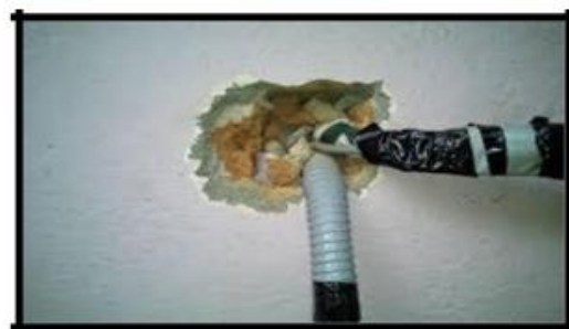
Figure.3. Tiles break while drilling.
