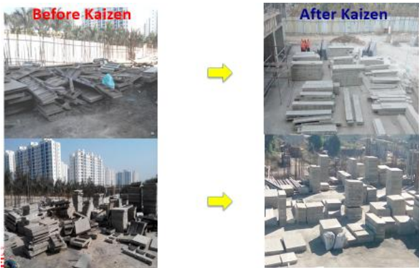
Figure.6. Before & After (Missing Aluform Shuttering found)
